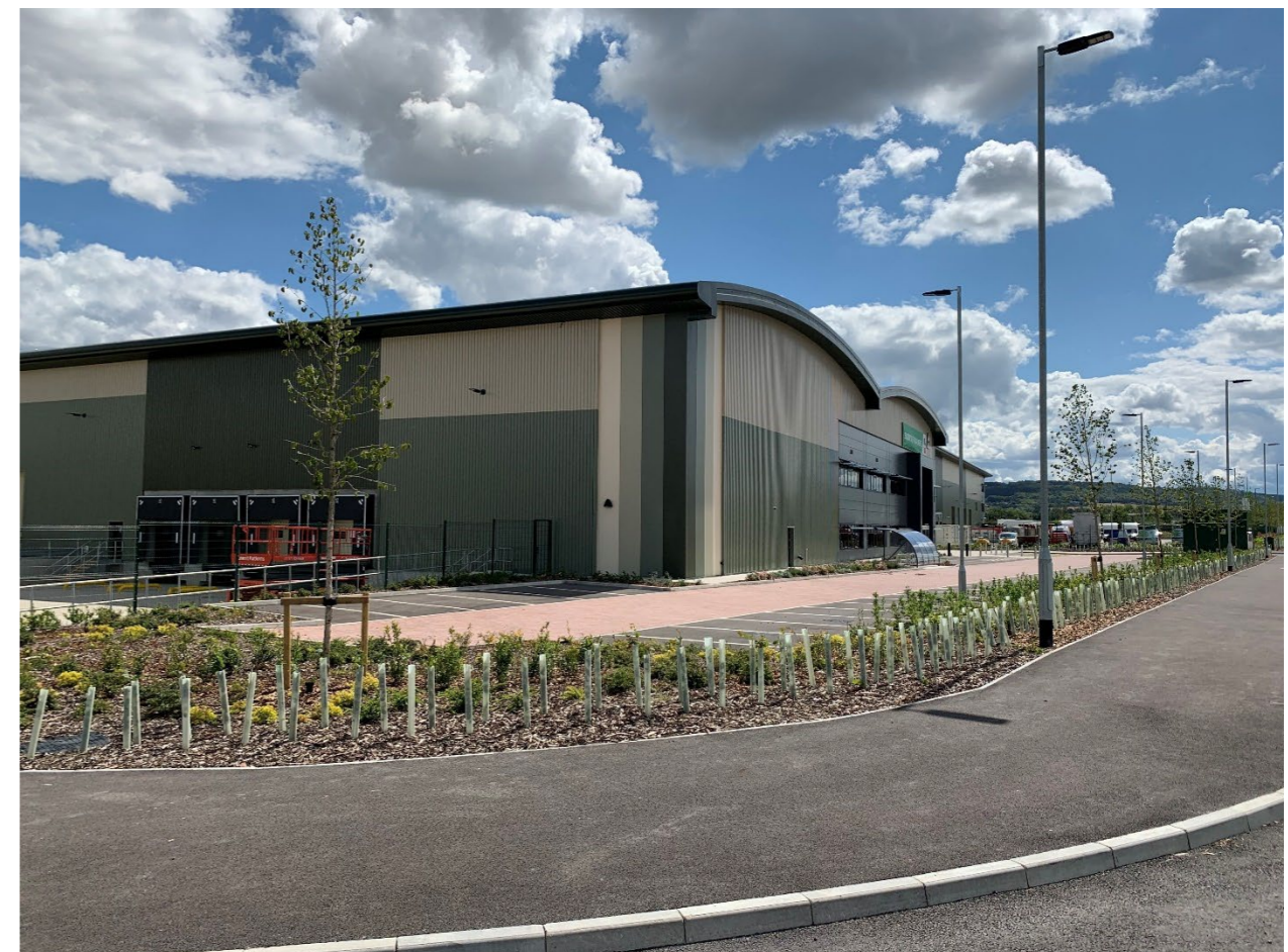
Fig 49. Column mounted and building mounted, light fittings for the development plots and highways.
